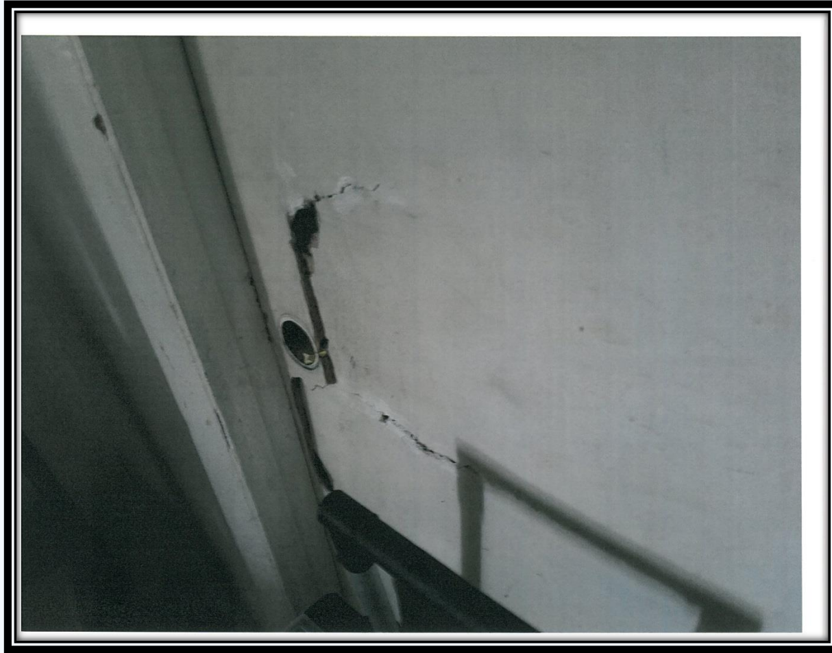
Missing door knob and damage
