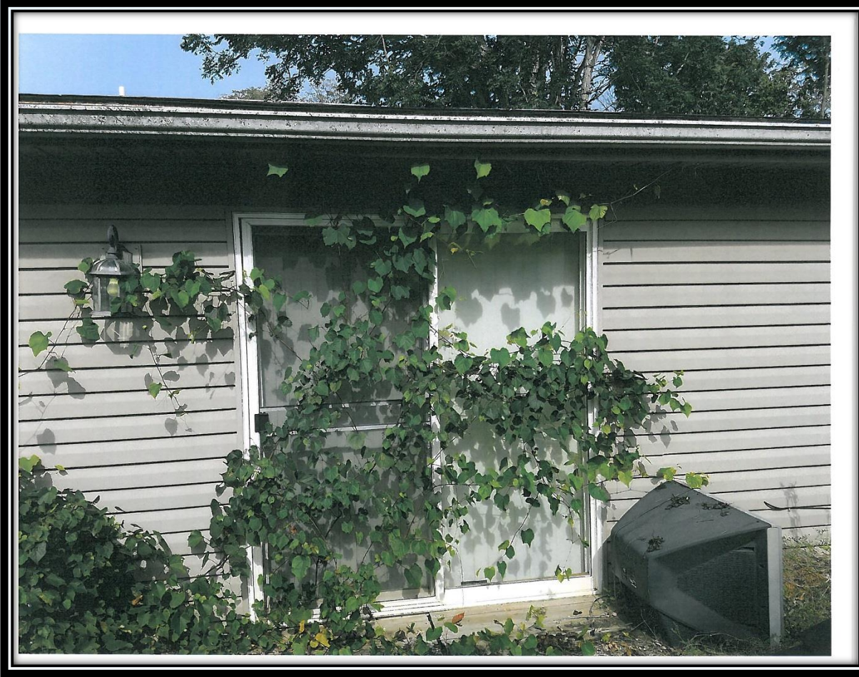
FIRE HAZARD Vines blocking an emergency exit
