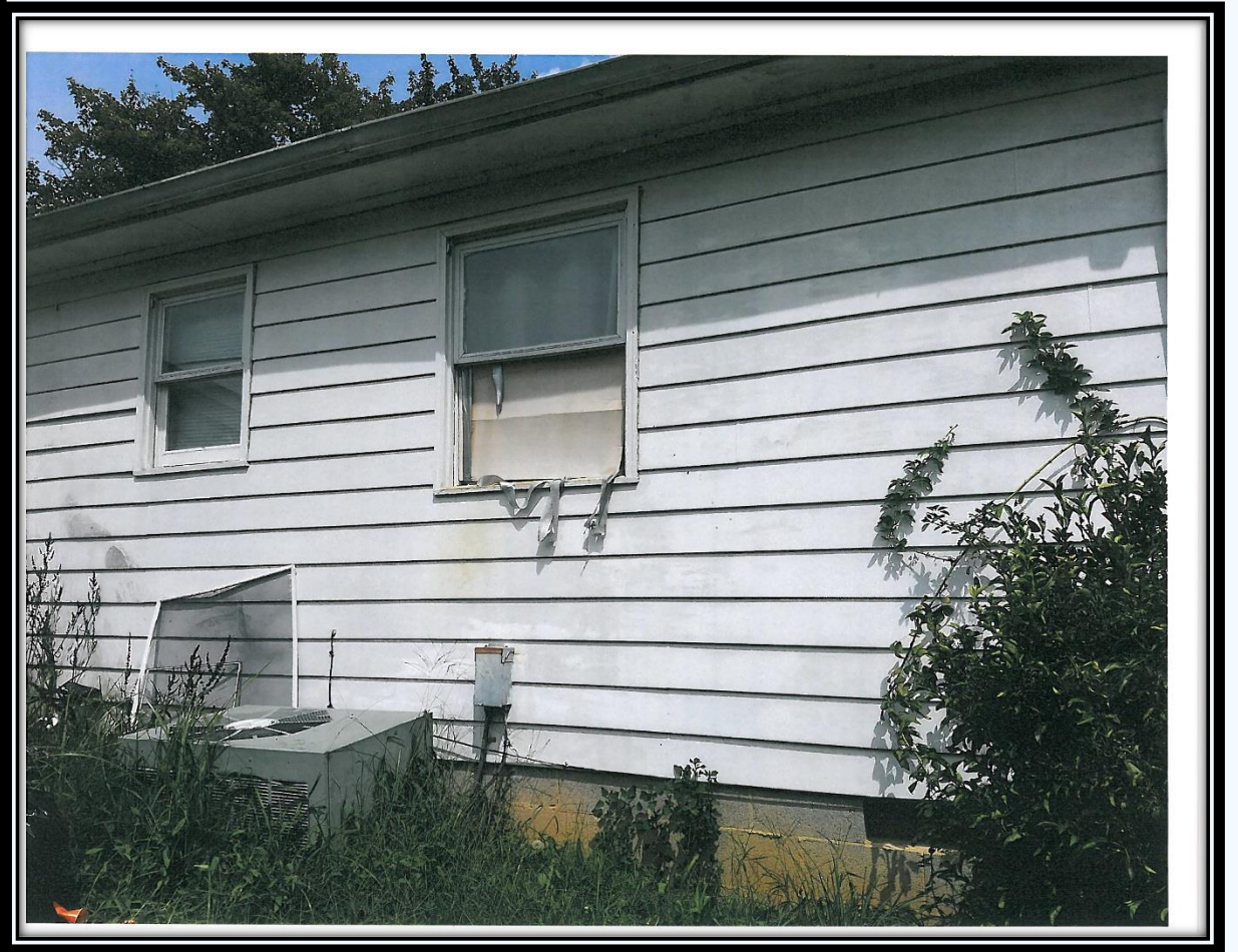
Missing bottom window pane
