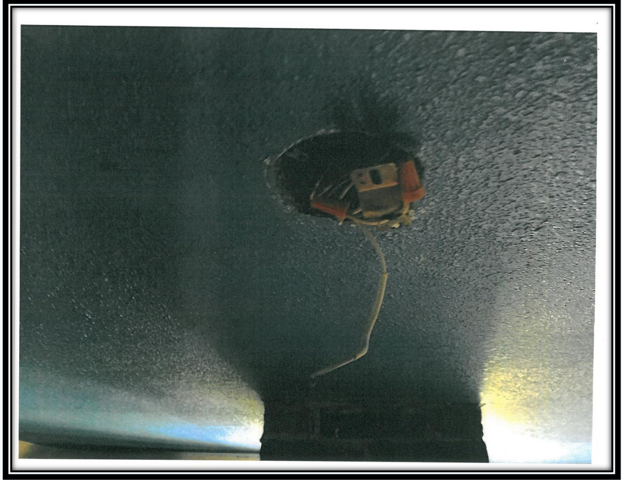
Missing Lighting Fixtures; Exposed Wires Hanging
