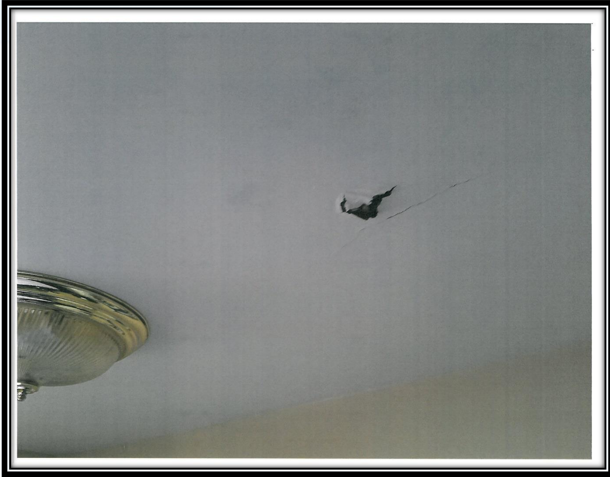
Hole in the ceiling
