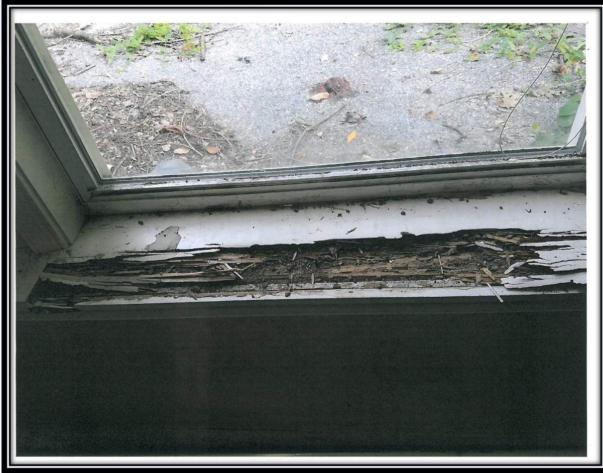
Damaged window sill
