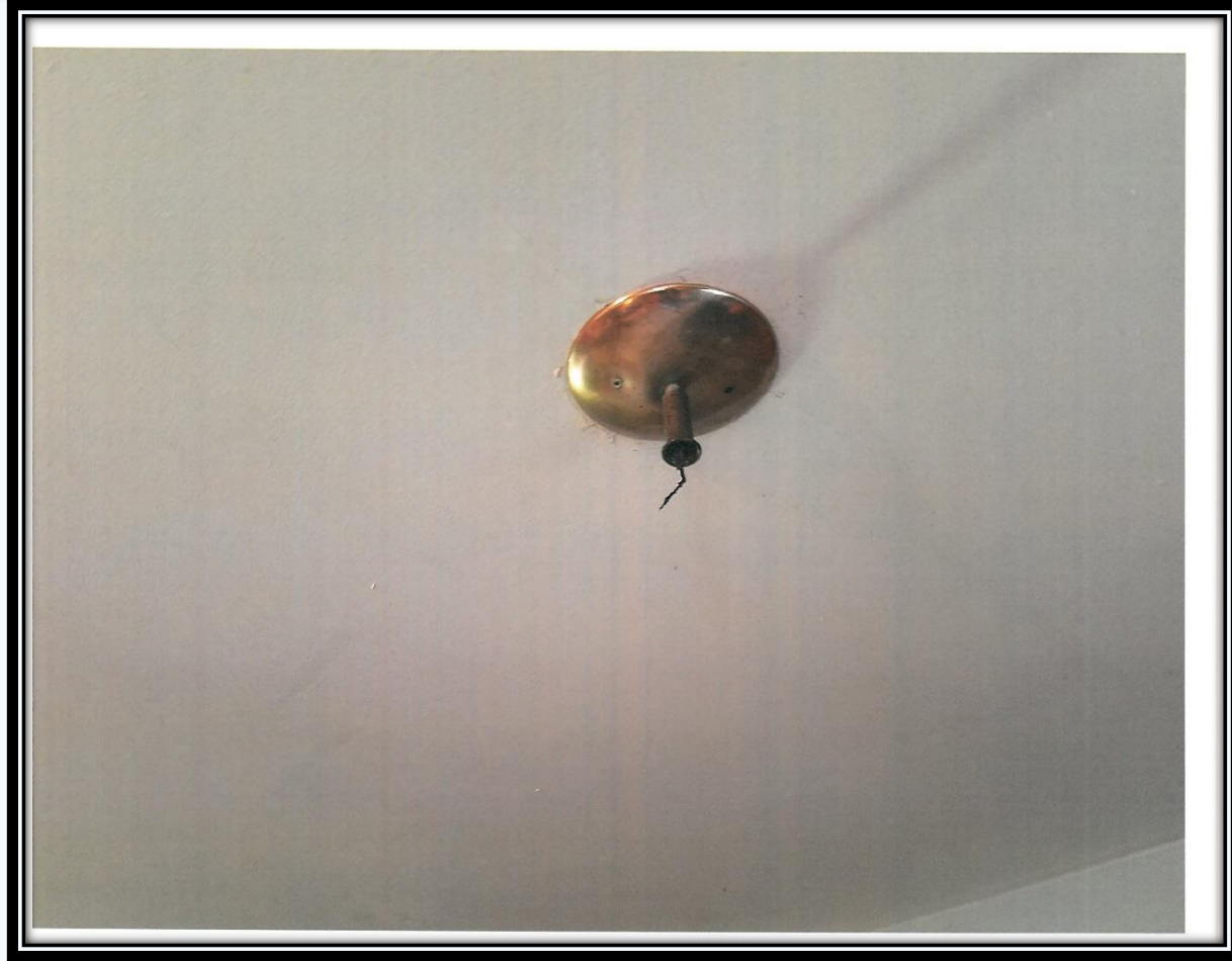
Missing Lighting Fixture; Exposed Wires
