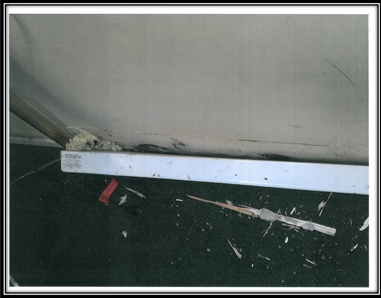
Secure and ensure that Electric Baseboard Heaters are in working order
