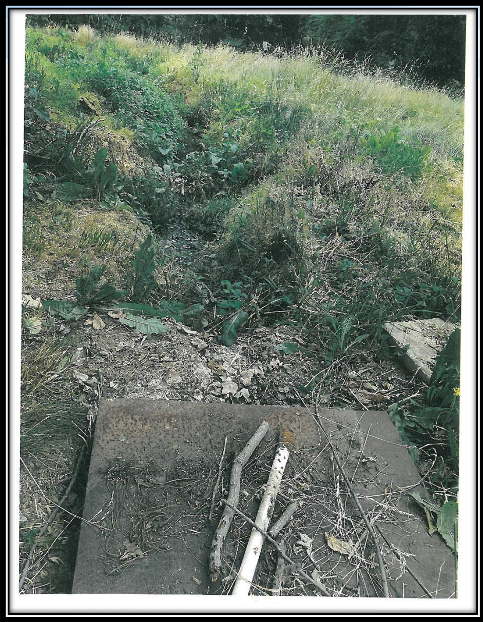
Septic tank issues
