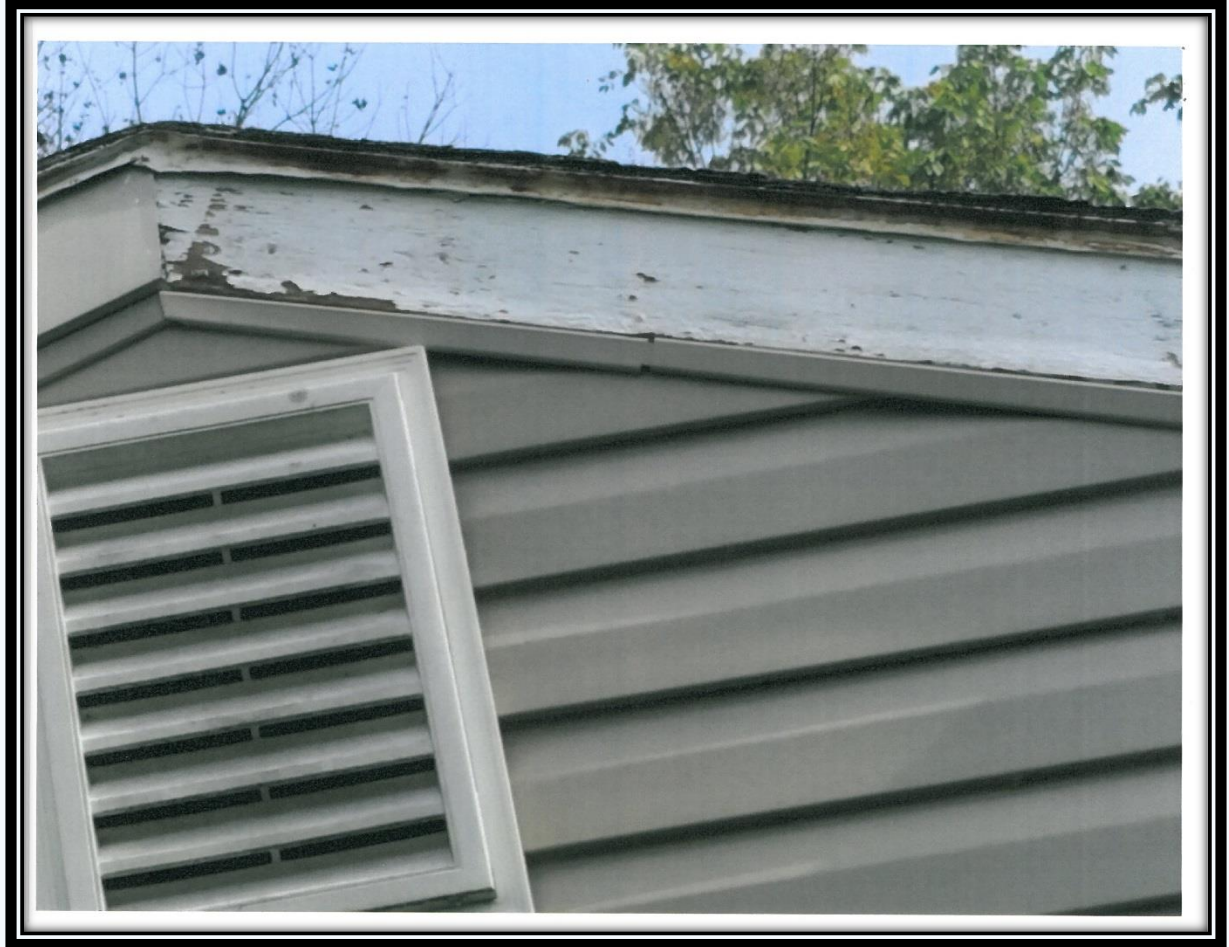
Vinyl siding peeling away
