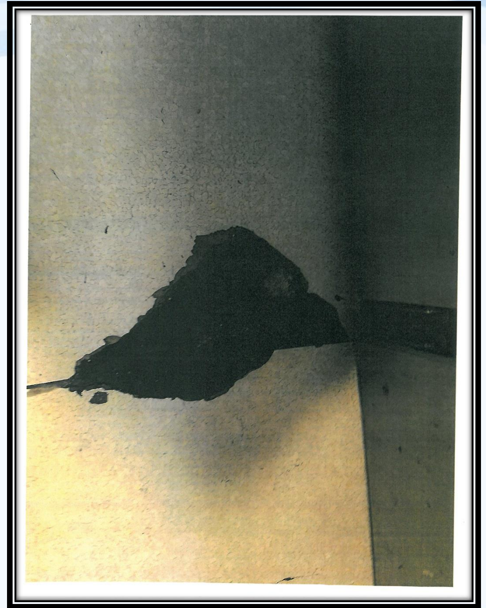
Vinyl flooring damaged
