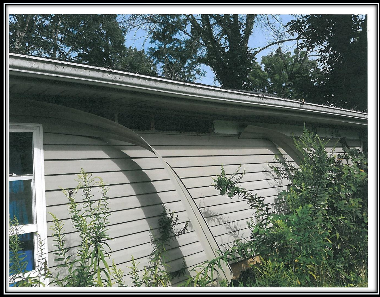
Vinyl siding peeling away
